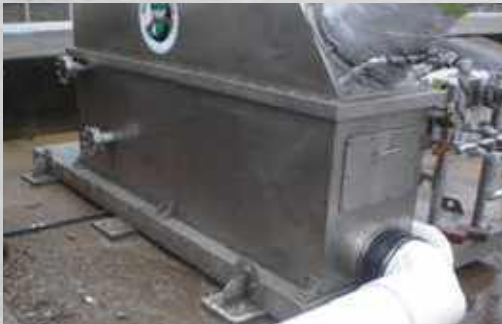
Skid Mounted System
