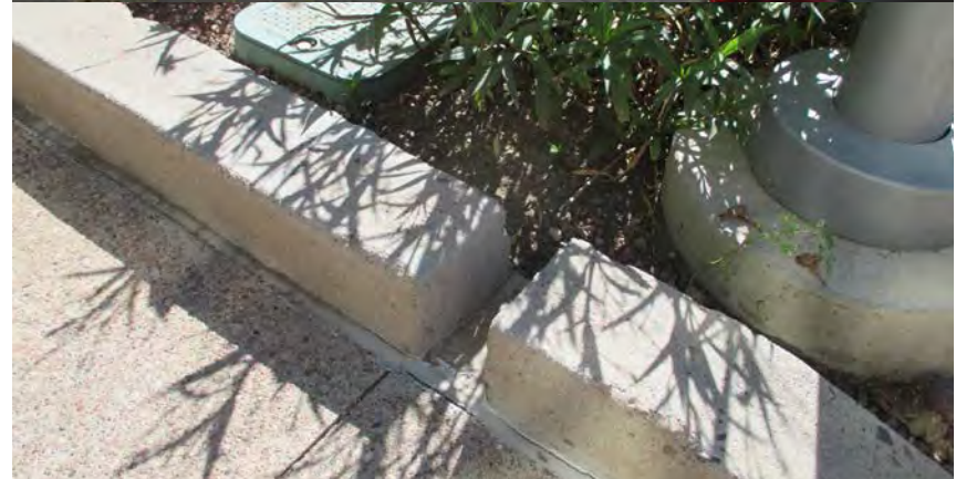
Standard curb cuts open up planting areas to receive stormwater flow.
