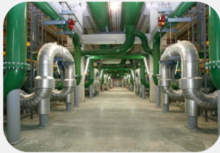
District Cooling Utility
