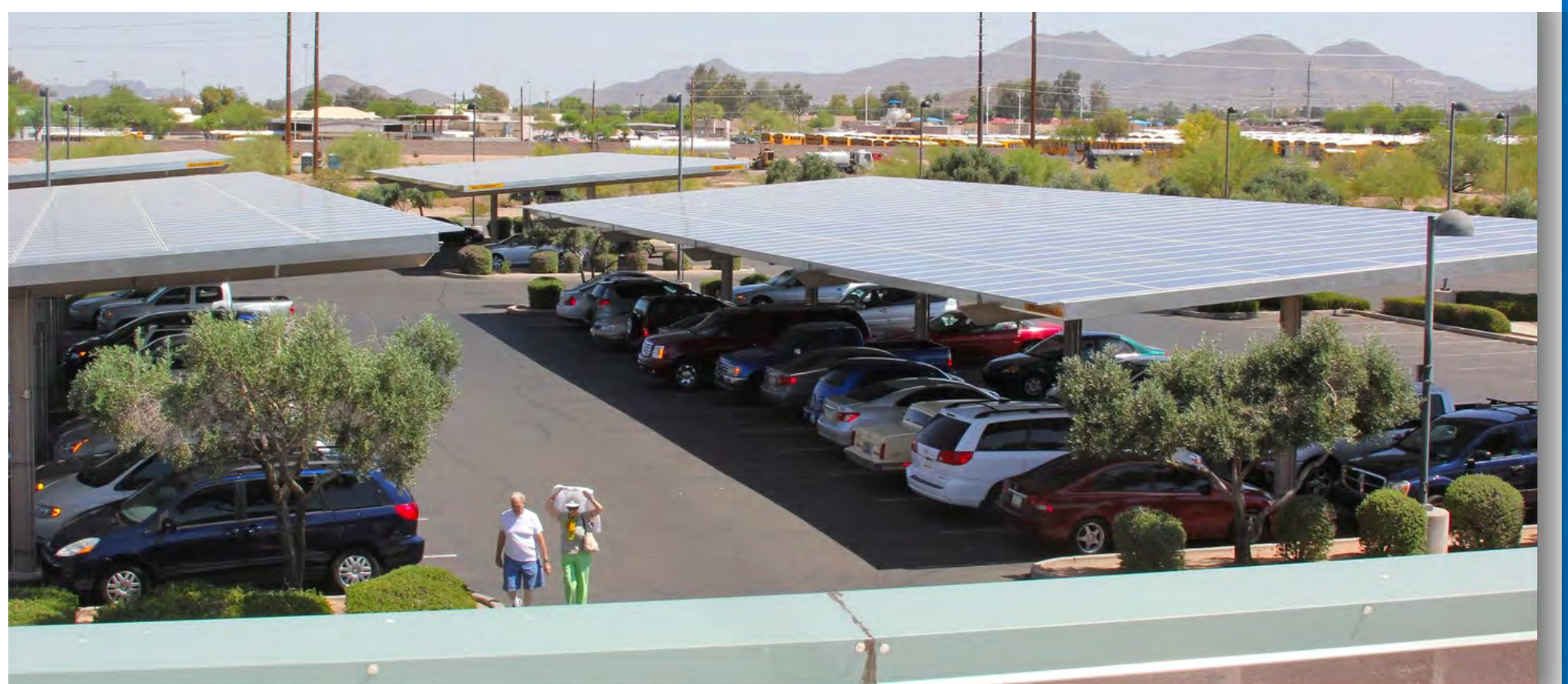
Red Mountain Library – 352 KW
