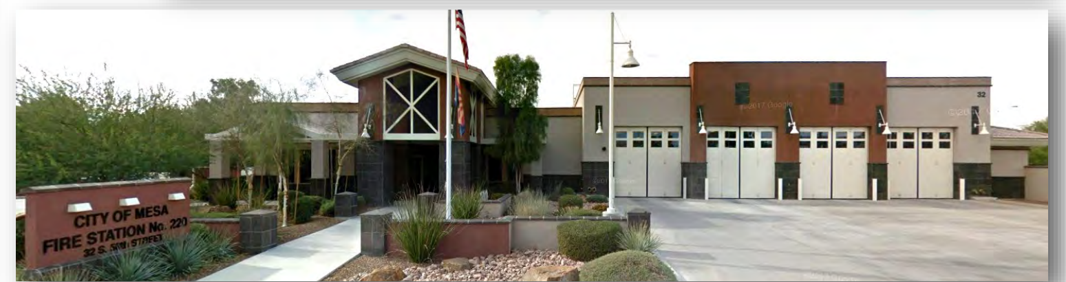
Fire Station 220 – 15 KW Photovoltaic Roof Mount
