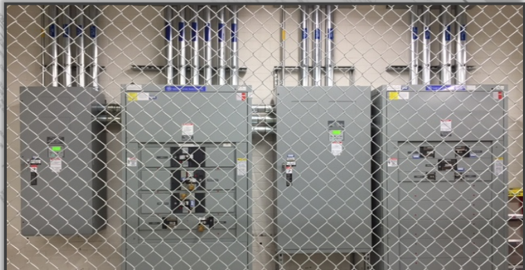
Communications Building Electrical/Mechanical
