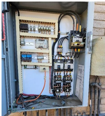
Figure 6 – Existing Bypass Pump Control Panel
