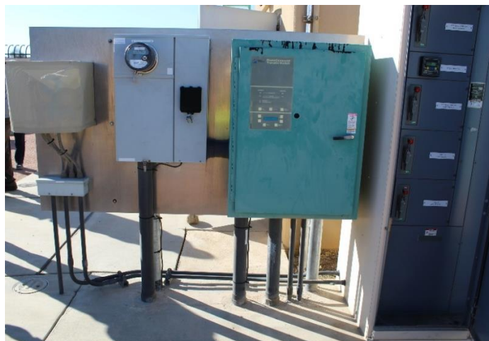
Figure 10 SES, ATS and Motor Control Center
