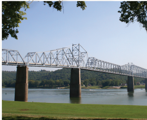
Milton Madison Bridge over the Ohio River between Kentucky and Indiana. Bridge projects can affect a variety of cultural and historic properties. (photo courtesy Wilbur Smith Associates/Michael Baker Engineers)
